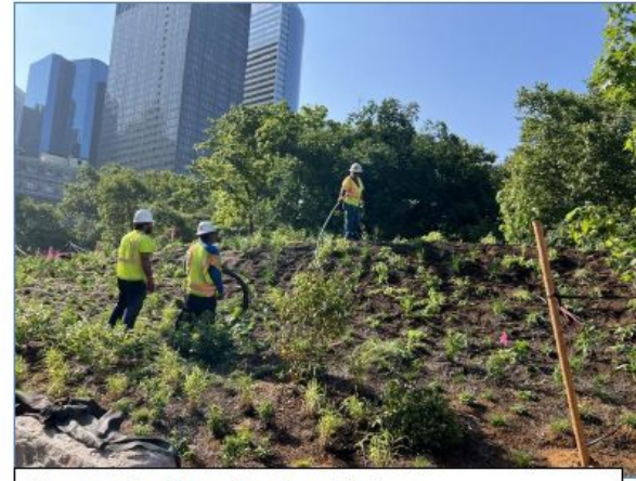
Battery landscaping installation
